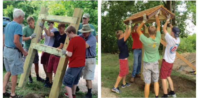
Madison Boy Scouts under the direction of SGT's Perry Rianhard built and erected a kiosk on the new section of trail.
