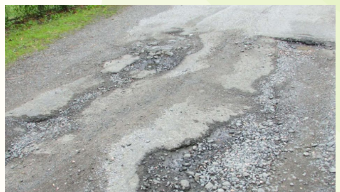
Asphalt damaged by the heat.
